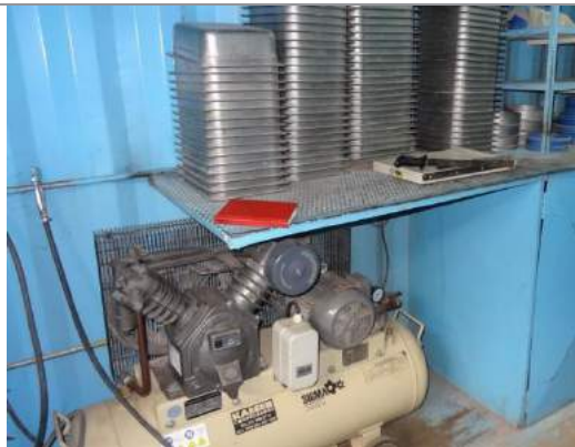
C Compressor and sample trays
