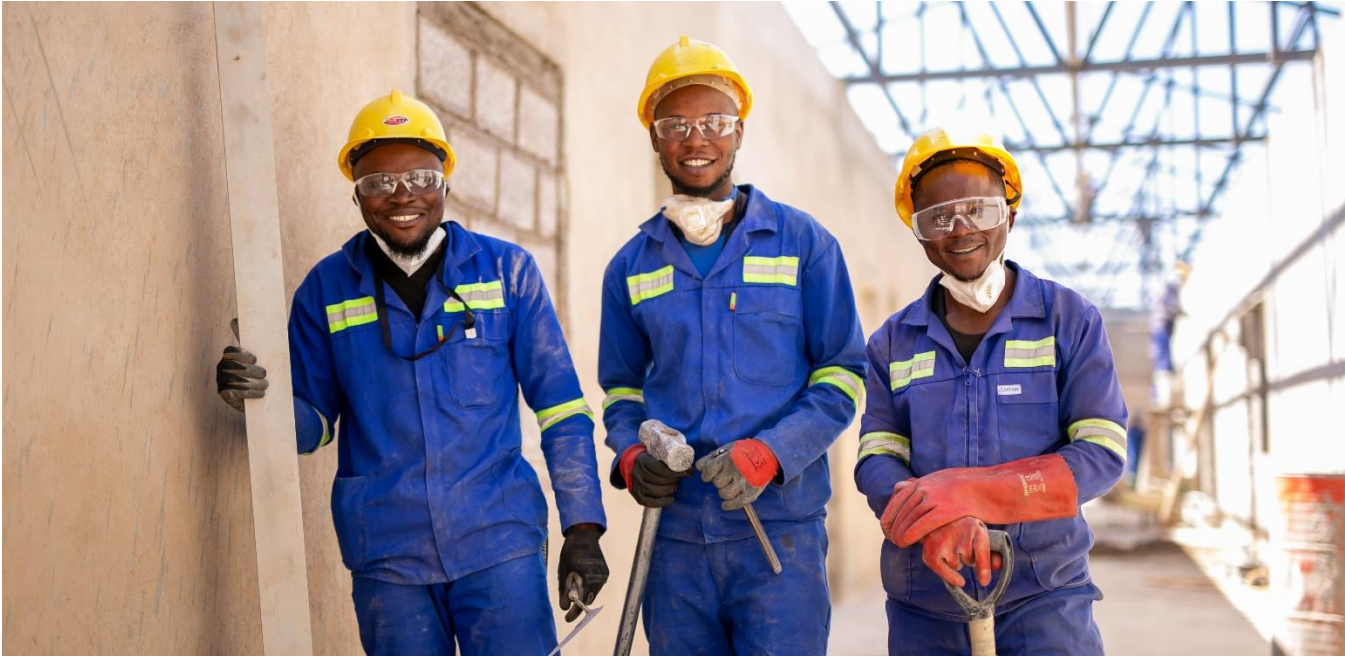
(L-R) Sipamba Mwamba, Kasaola Ilunga and Elie Ngoie Tshisola working on masonry at the new Kamoa hospital.
