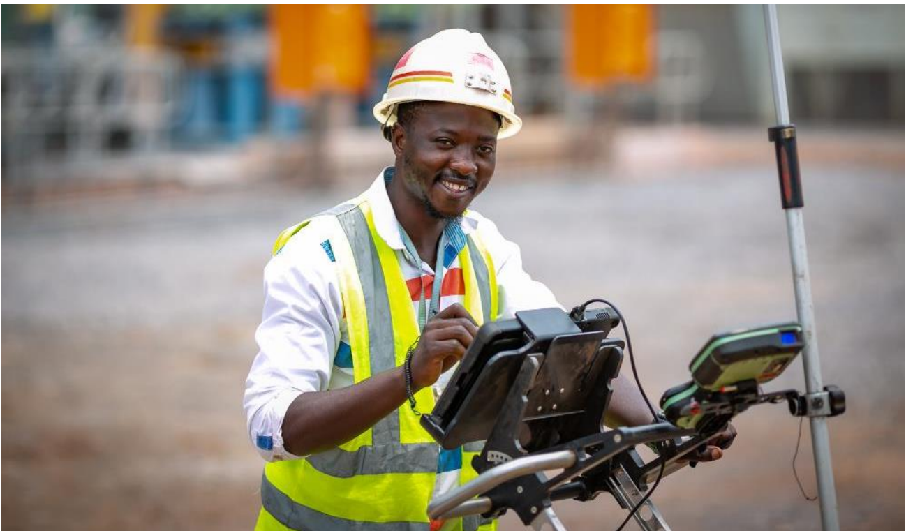
Surveyor Lumbu Ghislain Pansemoya using ground-penetrating radar to locate underground piping and cabling.
