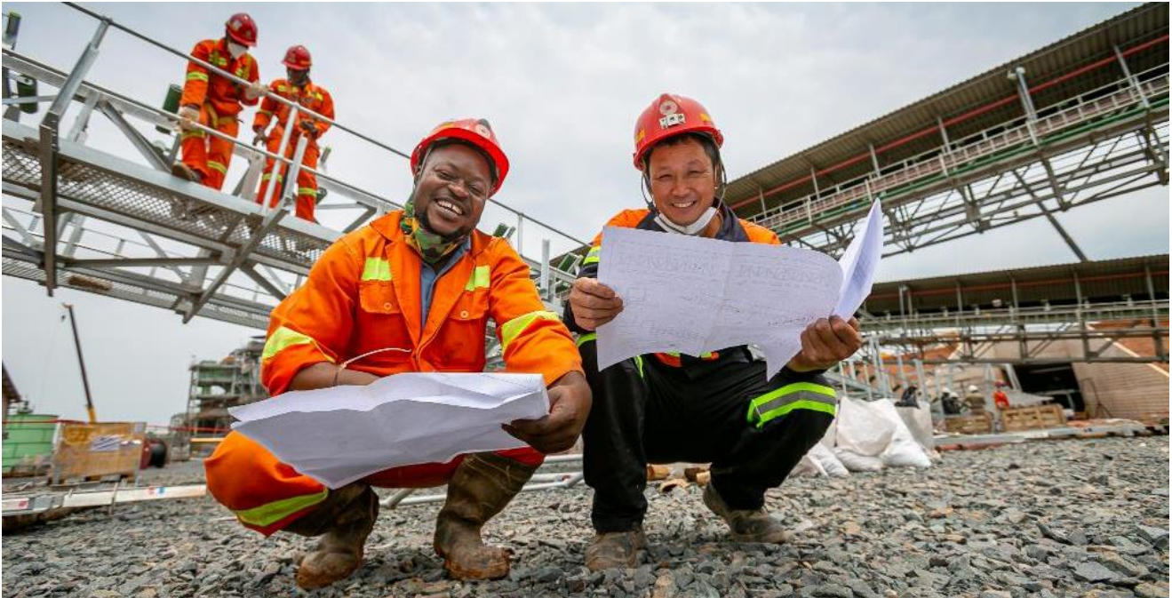
Wilbert Kakudji (left) and Jing Dong reviewing engineering drawings for the Phase 2 ore conveyor systems.
