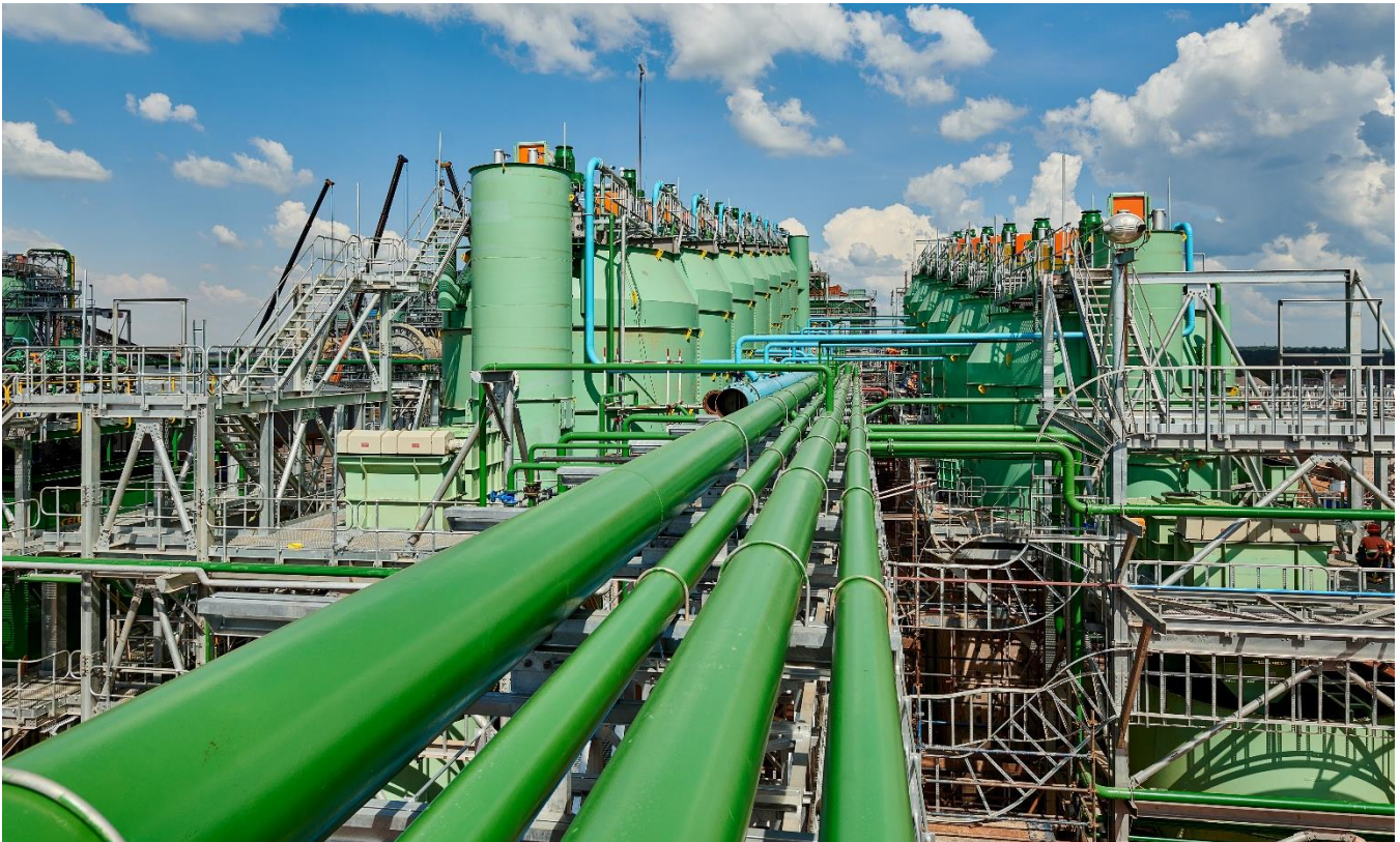
Installation of new piping for the Phase 2 flotation cells is progressing quickly.
