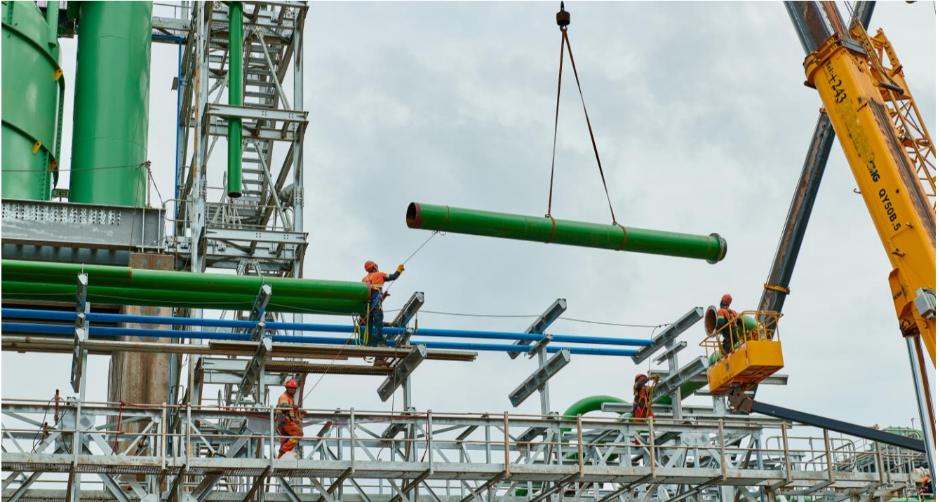
Crews lifting a section of piping into place for the Phase 2 concentrator.
