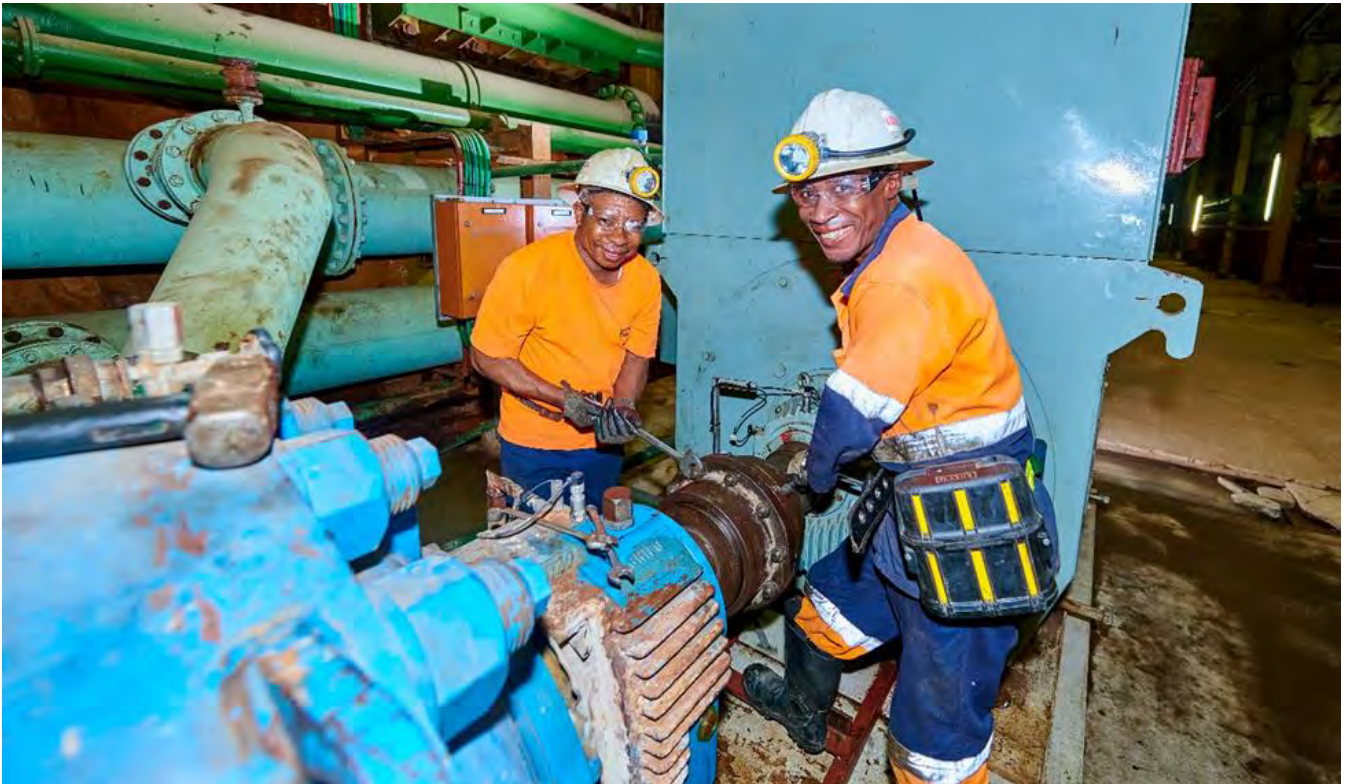
Photo: Mechanics Ndaye Ngoie and Banza Ngoie perform routine maintenance at Kipushi's 1,200-metre-level pump station.
